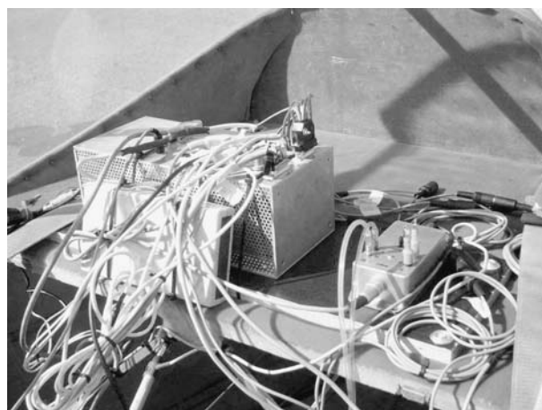
Figure 2 – Data acquisition box
